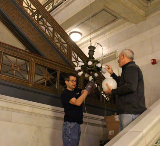
As part of Retrofit One, workers at the Cultural Center upgrade light fixtures with energy-efficient bulbs.
